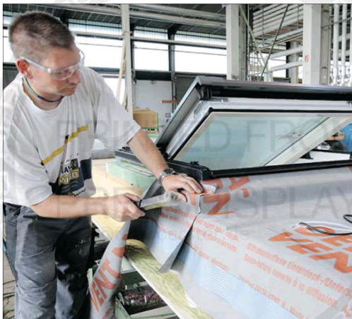
An employee installs a roof window into a pre-constructed section of a house at the Huf Haus GmbH factory in Hartenfels, Germany. Demand for factory-made houses is rising in Britain as homebuyers try to save money.
